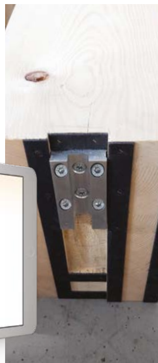
Strips of self-adhesive intumescent joint are laid around the connector and then stapled.
